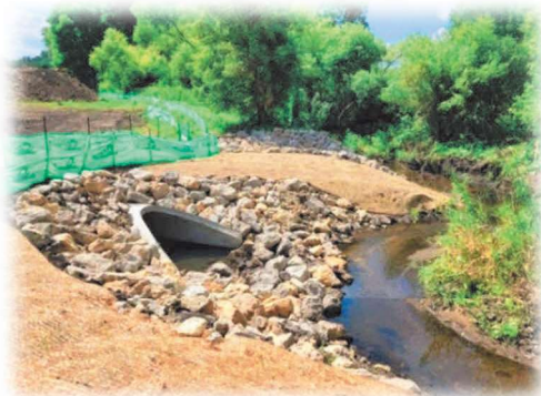
Figure E-5: Stormwater improvements on the North Creek tributary of the Vermillion River
