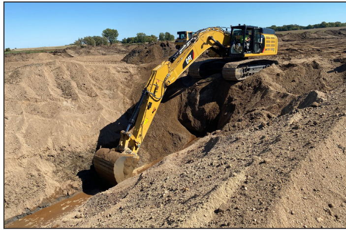
Contractor Tony Whitcomb of Atwater-based Tony Whitcomb Excavating dug a new channel for a Meeker County ditch in fall 2021 near Grove City as part of a wetland restoration on a 140-acre MN CREP easement site.
