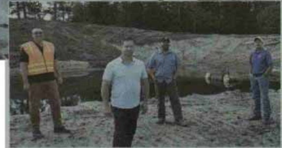
An iron-enhanced sand filter is part of the Beltrami County SWCD's Clean Water Fund-backed stormwater project designed to improve the water quality of nutrient-impaired Lake Irving, which flows into Lake Bemidji and then the Mississippi River. The stormwater project will keep an estimated 233 pounds of phosphorus out of Lake Irving each year. (Left to right): Zach Gutknecht, Beltrami County SWCD clean water specialist, checked on progress Sept. 9 in Bemidji with Tim Terrill, executive director of the Mississippi Headwaters Board; Shawn Tracy, HR Green lead scientist; and Chad Severts.
