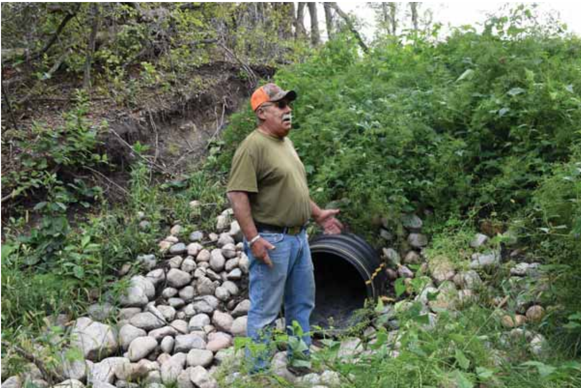
Joe Ste. Marie talked with Red Lake County SWCD staff about the improvements he's seen since a grade stabilization structure was installed at the edge of his Terrebonne Township field. A 30-inch-wide, 130-foot-long pipe now carries water from the field to this point, where it is filtered before reaching a Clearwater River tributary.
