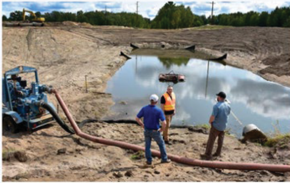
Zach Gutknecht, center, Beltrami County SWCD clean water specialist, visits the construction site of a stormwater treatment project on Sept. 9 in Bemidji with Shawn Tracy, right, HR Green lead scientist, and Chad Severts, SWCD board conservationist. An iron enhanced sand filter is part of the Clean Water Fund-backed stormwater project designed to improve the water quality of nutrient-impaired Lake Irving. The work will keep an estimated 233 pounds of phosphorus out of Lake Irving each year. (Courtesy / Ann Wessal)
