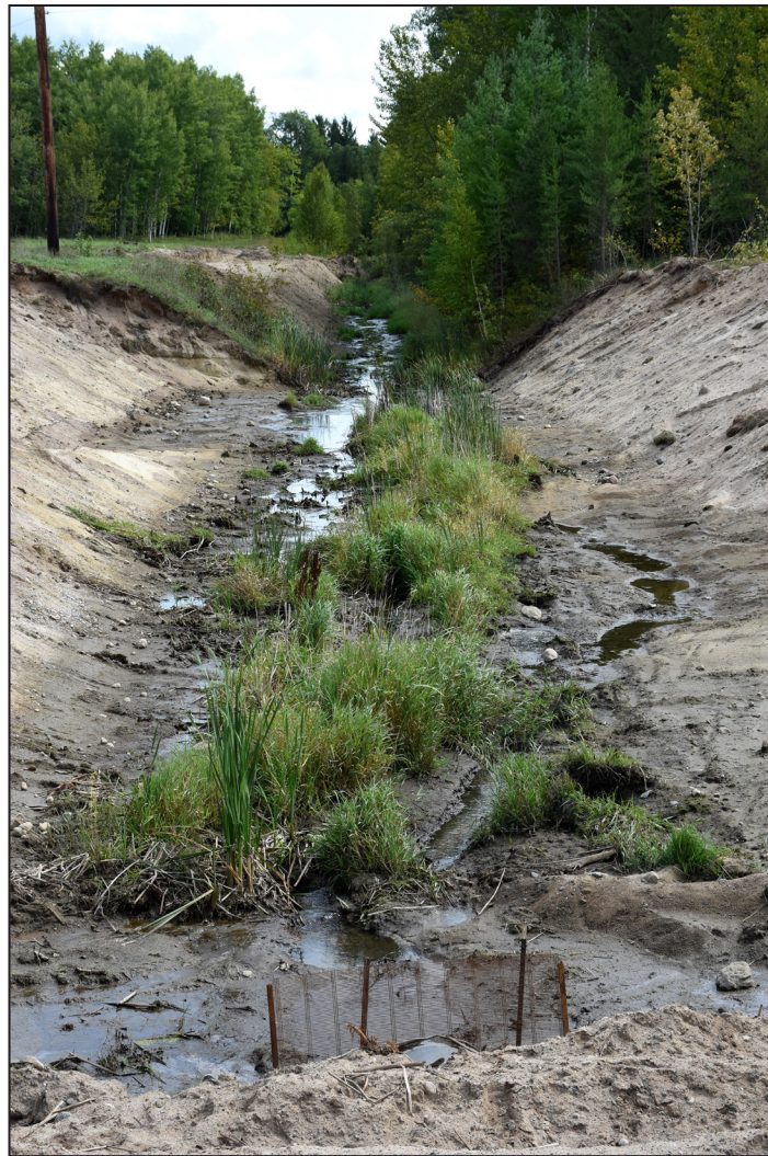
The Lake Irving ditch is being re-meandered to look and function more like a stream. It’s part of the Beltrami SWCD’s Clean Water Fund-backed stormwater treatment project, which is designed to benefit nutrient-impaired Lake Irving and estimated to keep 233 pounds of phosphorus out of the lake each year.
