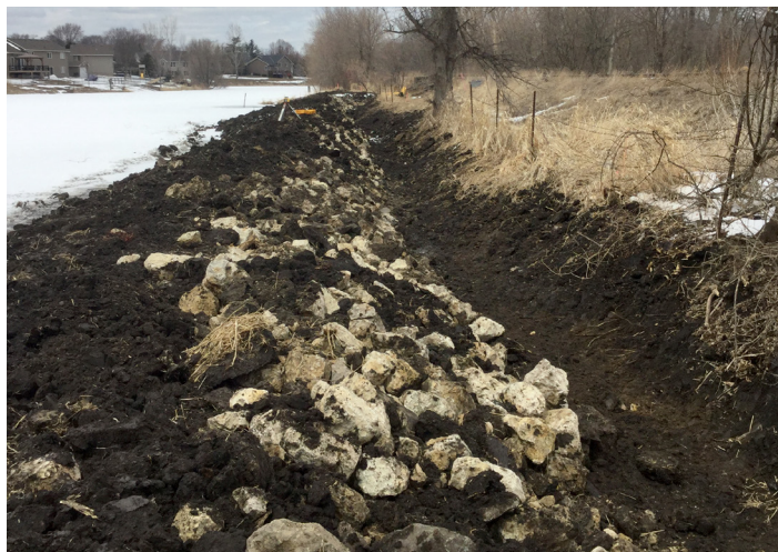
Vegetated riprap helps to stabilize the streambanks and control erosion. Photo Courtesy of Lakeville city staff
