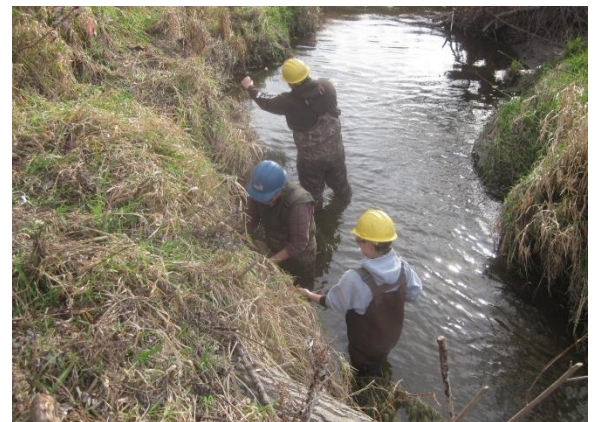
Live stakes are installed as part of a project with the Conservation Corps of Minnesota and Iowa.
