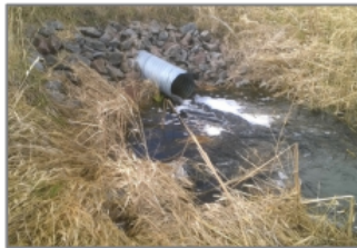
Figure 1. Upstream Drainage Tile Outletting into Restored Wetland
