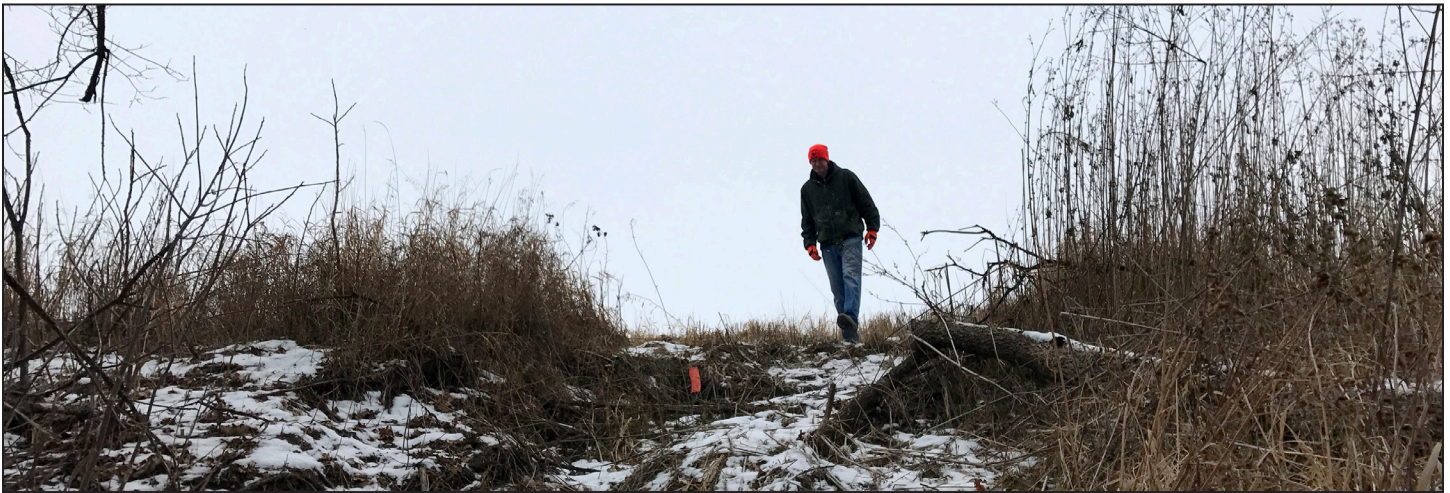
Wright SWCD Manager Luke Johnson leaves the field at a spot where water had carved a gully, which extended through an RV park.
