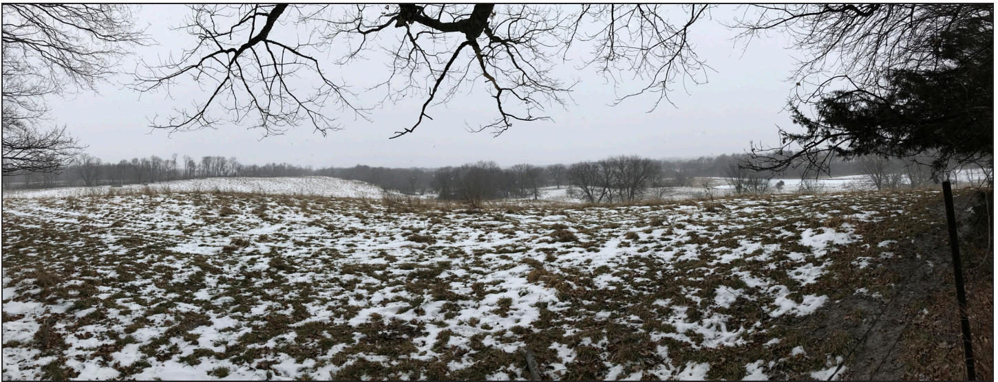
In the first phase of a three-phase project, Wright SWCD in 2013 installed two large grade-stabilization structures — one drains about 40 acres, the other about 15 acres — to fix a gully that was delivering sediment into the North Fork Crow River. The land is seen here from a county park; the distant treeline marks the river.
