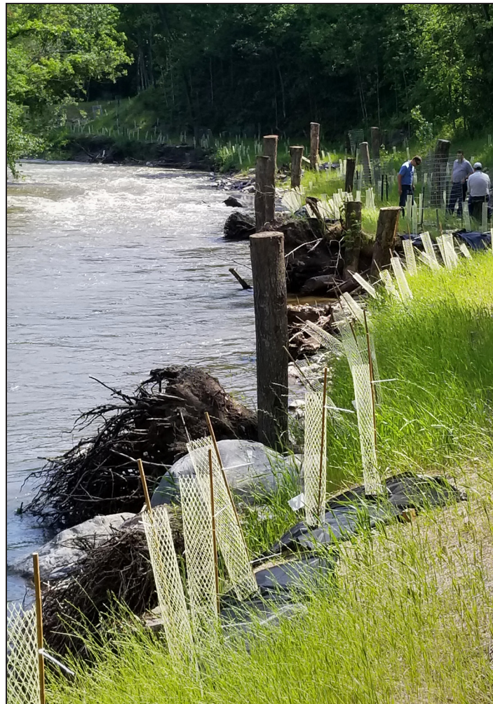
From left: Ryan Holzer, Scott County water resources scientist, views the Sand Creek bank stabilization project with Troy Kuphal, Scott Soil & Water Conservation District director, and Paul Nelson, Scott County environmental services program manager, on June 13 near Jordan.
