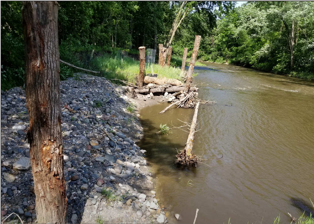
Between the root installations are a series of bays. The project is seen from farther downstream.
