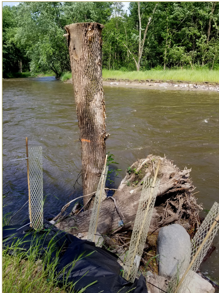
Bolts hold tree trunks and roots in place along a bend in Sand Creek, where fast-moving water has caused erosion.
