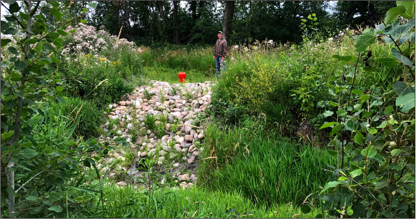
Torin McCormack, Roseau River Watershed District specialist, puts into perspective the size of a grade stabilization structure bordering Tony Brateng's fields on Aug. 2 south of Roseau. Contractors removed trees, resloped the ditch banks and lined them with fabric and rock where erosion once cut away at the field and sediment once entered the creek that empties into the Roseau River. Photo Credits: Ann Wessel, BWSR
