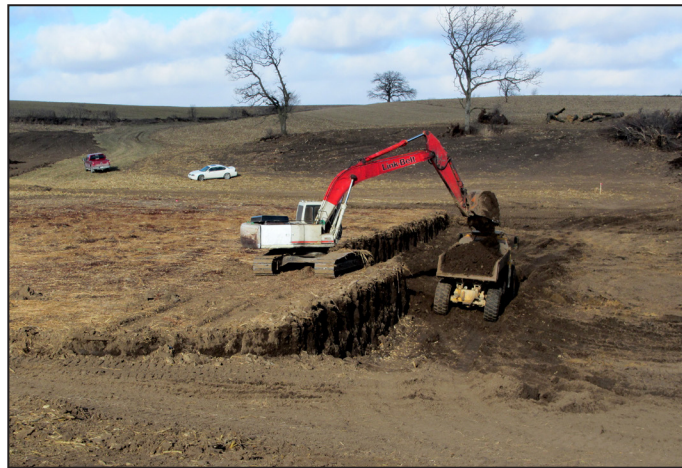
Top: Adam Beilke, BWSR board conservationist, and Donna Rasmussen, Fillmore SWCD administrator, talked Sept. 8 as they viewed the East Willow Creek Flood Control Project rehabilitation site. Photo Credit: Ann Wessel, BWSR
