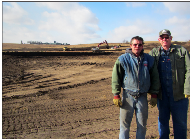
Mark Mensink, left, and Rick Mensink, checked progress of work Dec. 5 on their land southwest of Preston. Their grandfather, Art Mensink, allowed construction of the initial East Willow Creek Flood Control Project. After the sediment pool filled in, the Mensink brothers said their father, John, had farmed the 3-acre site.
