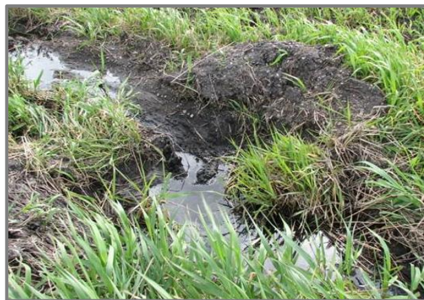
Figure 11. Eroded Channel above Settled Tile Block Trench
